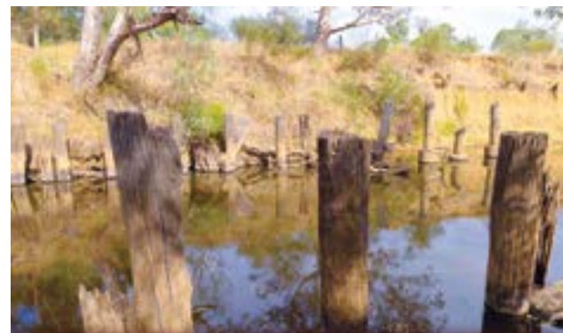
Remnants of the Jenkin Bridge over the Loddon River @ Newstead, 2 February 2025.
